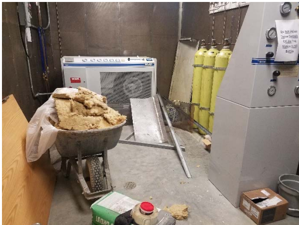
Photograph 63. View of the room used to fill air tanks.
