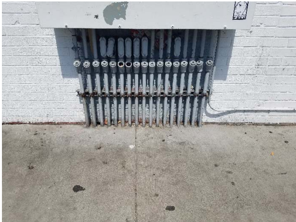
Photograph 27. View of the UST tank valves and electrical hookups.
