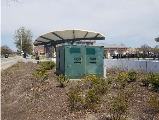
Photograph 41. View of the western structure associated with the HRT bus terminal and pad-mounted electrical equipment.
