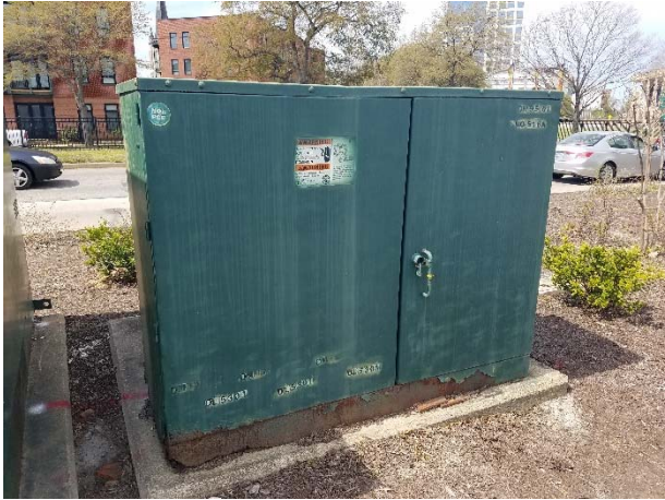
Photograph 42. View of the non-PCB pad-mounted electrical transformer.
