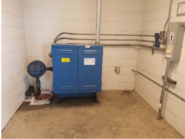
Photograph 57. View of within the elevator room. Note the staining on the floor from leaking fluid and drip pan.
