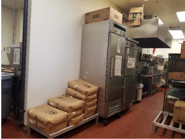
Photograph 13. View of the food storage and cooking prep areas of the kitchen.
