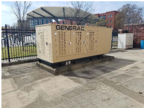
Photograph 51. View of the emergency generator located in the southern portion of the property.
