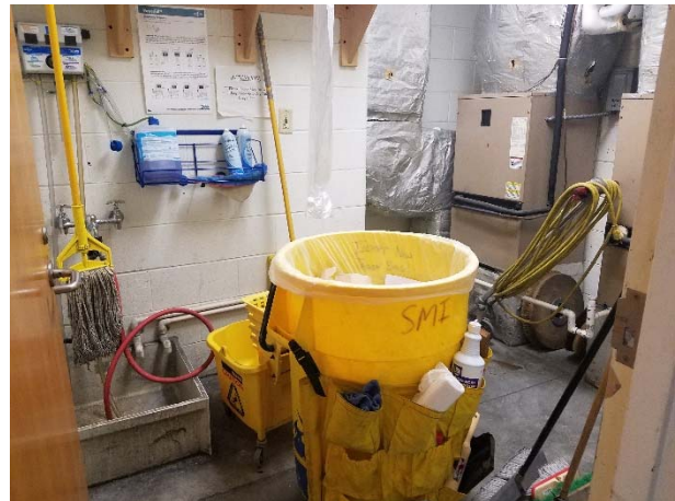
Photograph 64. View of a representative utility closet within the building (first floor).
