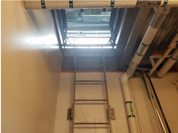
Photograph 48. View of the ladder access to the ventilation system and roof within the utility closet.
