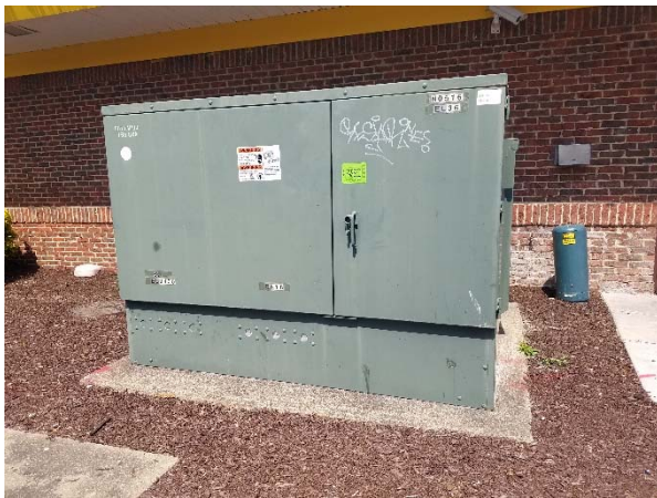
Photograph 19. View of the Non-PCB, pad-mounted electrical transformer located on the south side of the building.
