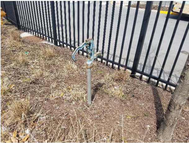
Photograph 29. View of the lawn hydrant located along the northern property boundary.
