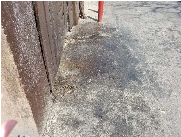
Photograph 7. View of the grease staining.
